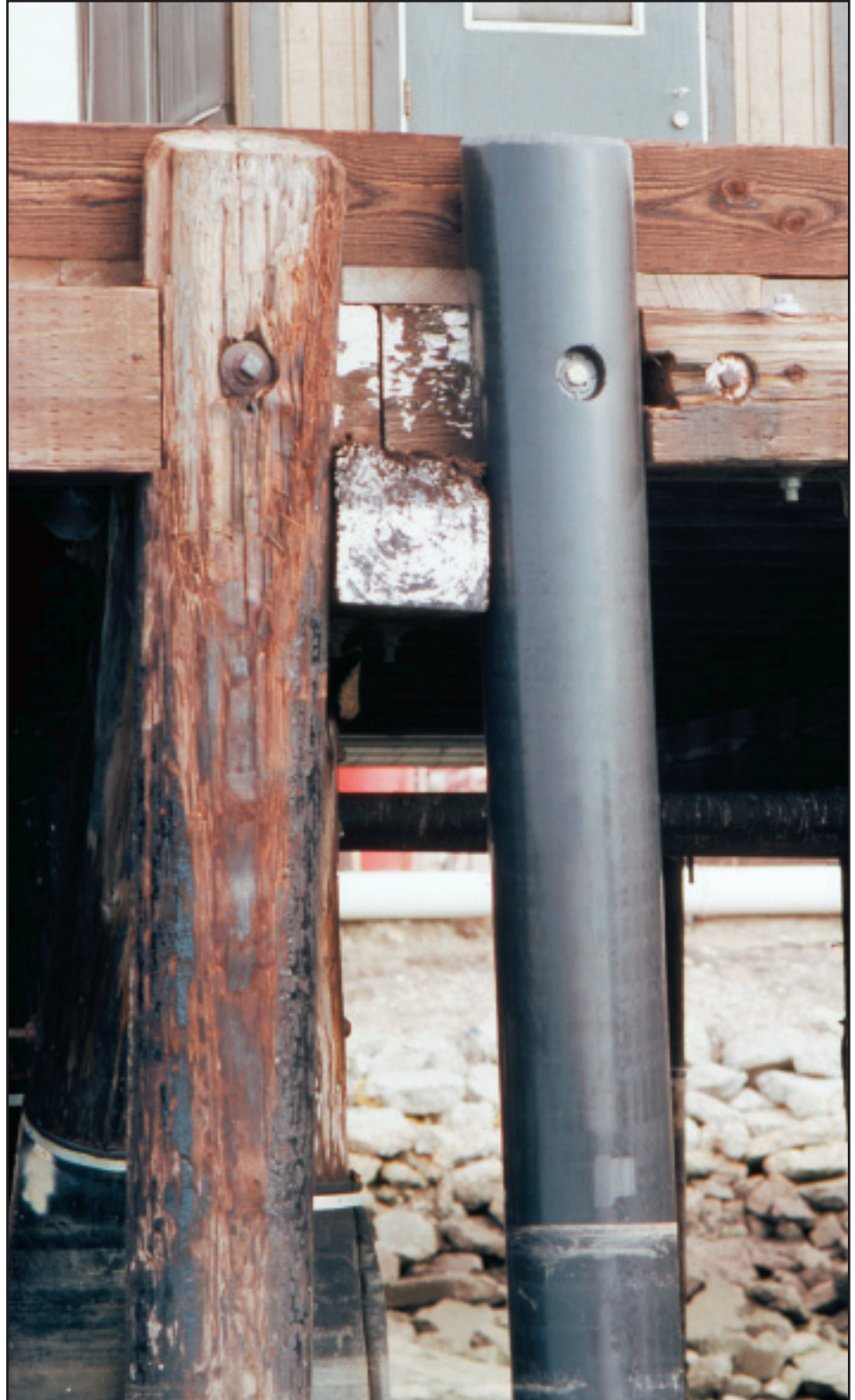
SEAPILE Composite Marine Piling installed as a replacement to a traditional wood fender pile at a large oil tanker terminal.
